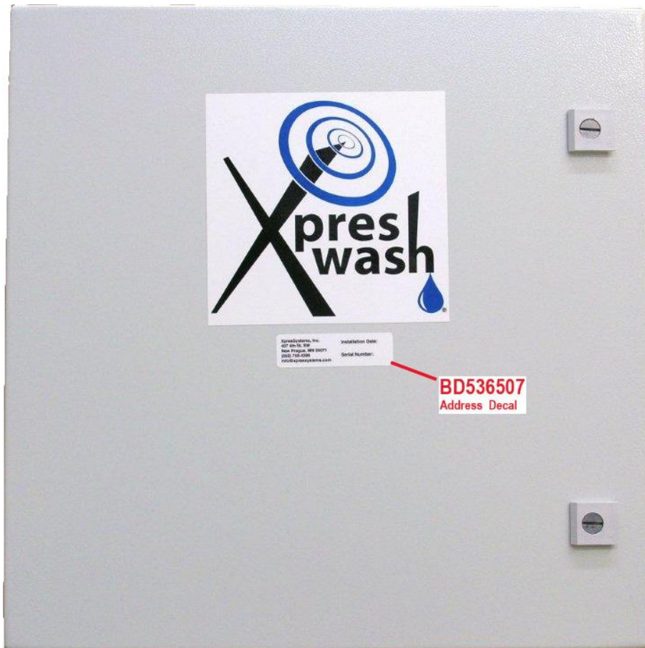
Figure 8: Computer Cabinet External Misc Components
